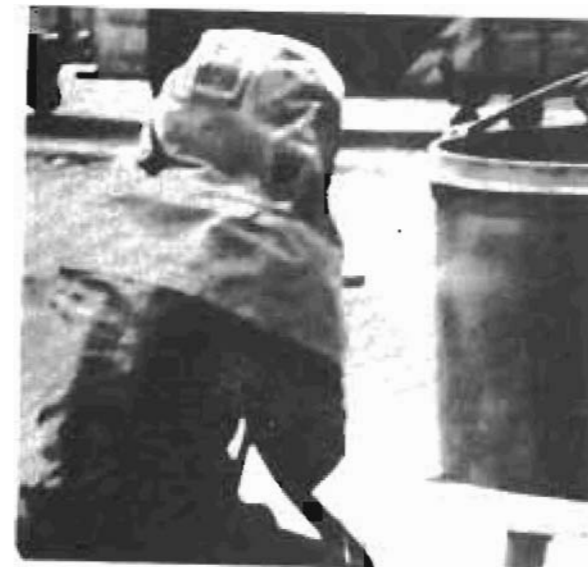
Figure 23 - An Inadequate Ricochet Hood for Sandblasting
