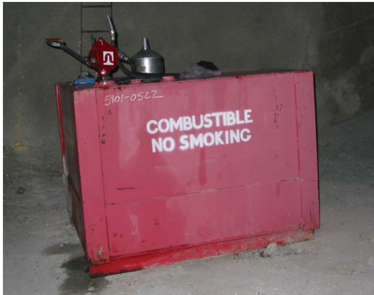
Figure 8.—Fueling station in isolated zone.
