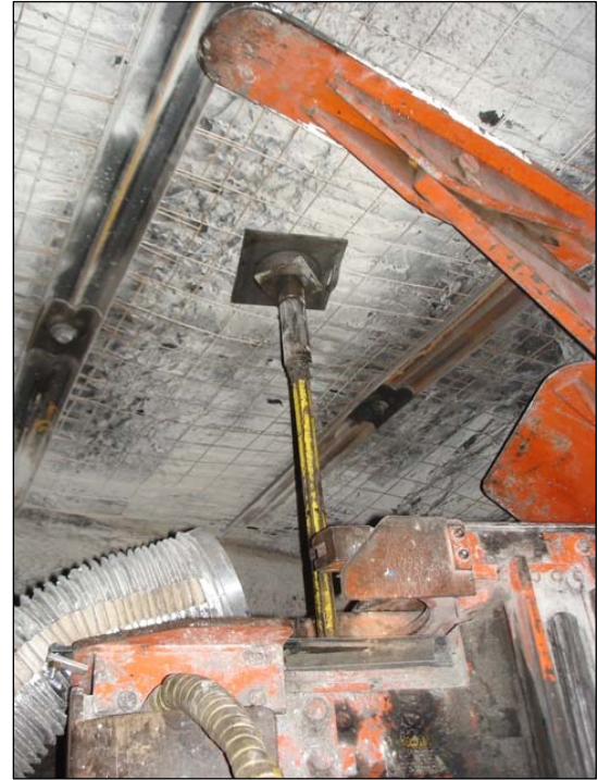
Figure 4.—Once drilling is completed, the CDSE is moved aside so the roof bolt can be installed.
