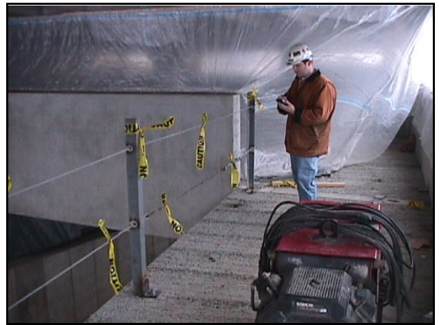
A WVU Fall-Safe coordinator audits a guard rail at a Fall-Safe contractor's site.
