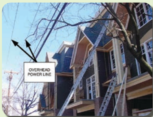
Figure 1. Overhead power line 16 feet from the painting operation in FACE Case Study 2. Photograph courtesy of the North Carolina Occupational Safety and Health Administration [NIOSH 2004b].
