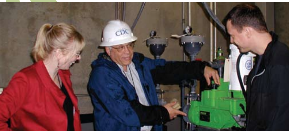
Kip Duchon, CDC's National Fluoridation Engineer with the Division of Oral Health, demonstrating the use of a chemical feed pump to add fluoride to community water supplies
