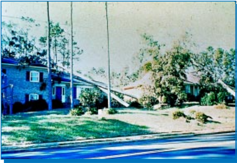
Hurricane Hugo wind damage, Charlotte, NC/NOAA
