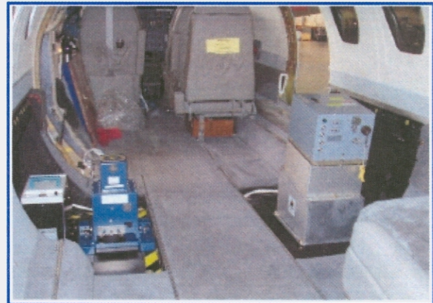
Figure 2: The Itres CASI-2 hyperspectral imager, Emerge/Applanix Digital Sensor System (DSS), and an Optech ALTM 2050 system installed on the NOAA citation aircraft (left to right). Click on image to see enlarged.
