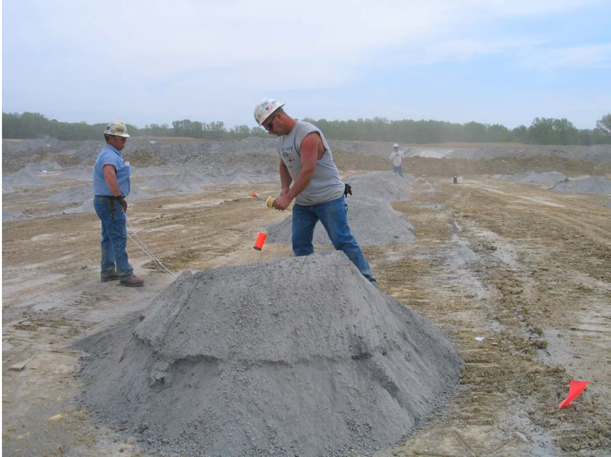
Figure 13 - Lowering a booster with an Orica I-KON™ electronic detonator into a blast hole
