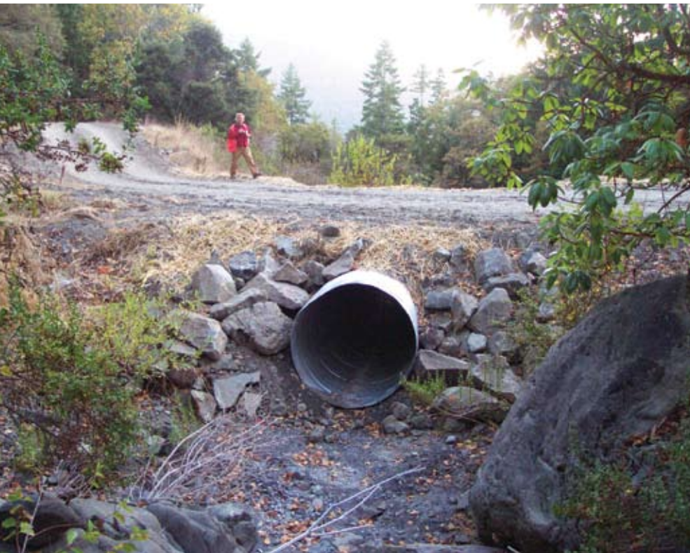
During restoration of Coyote Creek basin, the National Park Service and its cooperators installed new, larger-diameter culverts at stream crossings. The old culvert at this crossing was severely rusted and substantially undersized for even moderate winter storm flows. The new culvert is 60 inches (150 cm) in diameter, which is large enough to accommodate a 100-year flood.
