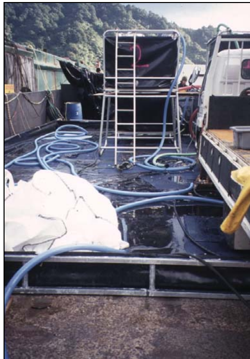
Figure 9. The entire filtering system was contained inside a 300 mm high sealed cofferdam made of 1 mm thick impermeable polypropylene (Ultraflex) to contain any spillage or overflow during the vacuuming operation. Photo courtesy of New Zealand Diving and Salvage Ltd.
