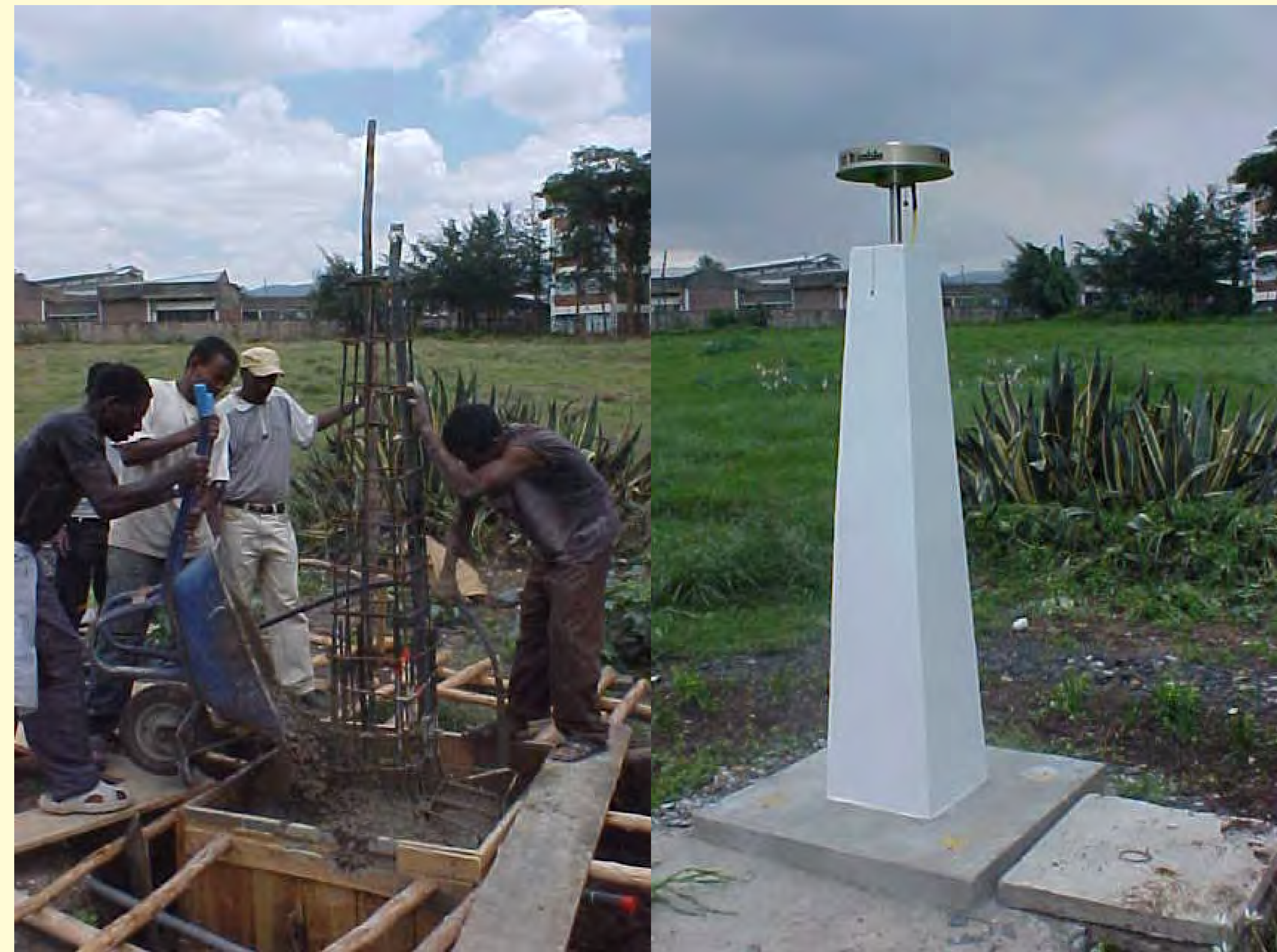
Monumentation and initial installation of IGS station ADIS with GNSS antenna
