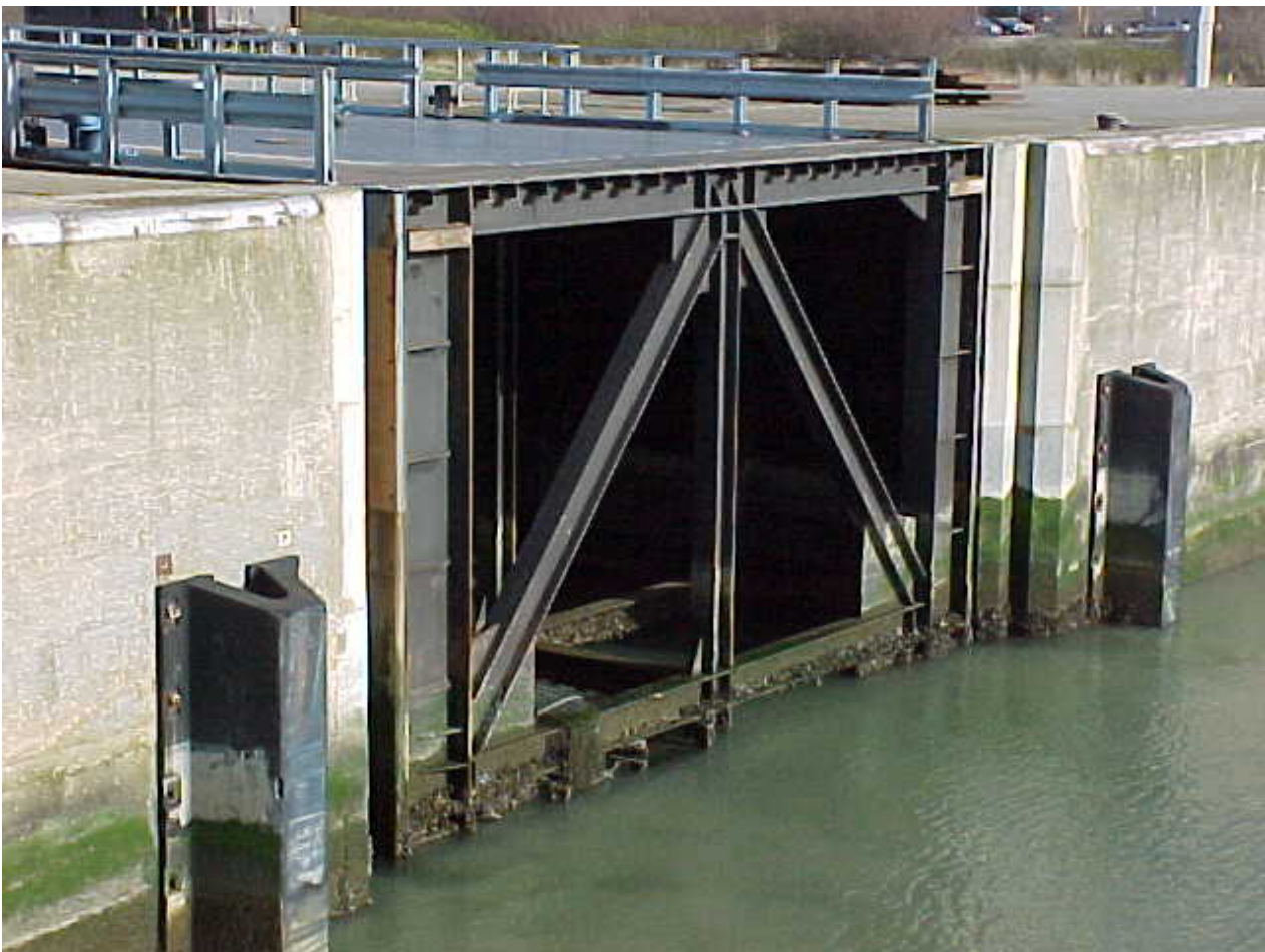
Picture of a rolling gate in its recess in the P. Vandamme lock in Zeebruges – Belgium
