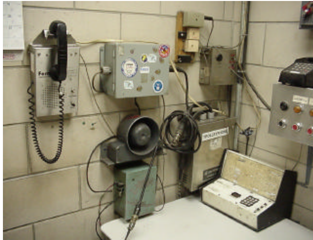
Example of a communication station for dispatcher
