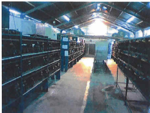
Typical Lamp room with battery charger racks
