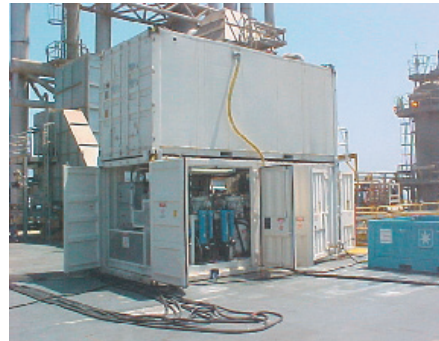
Nitrogen generator on a gas lift in Qatar
