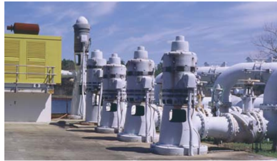
Figure 18. Public supply water intake in Bay County, Florida.
