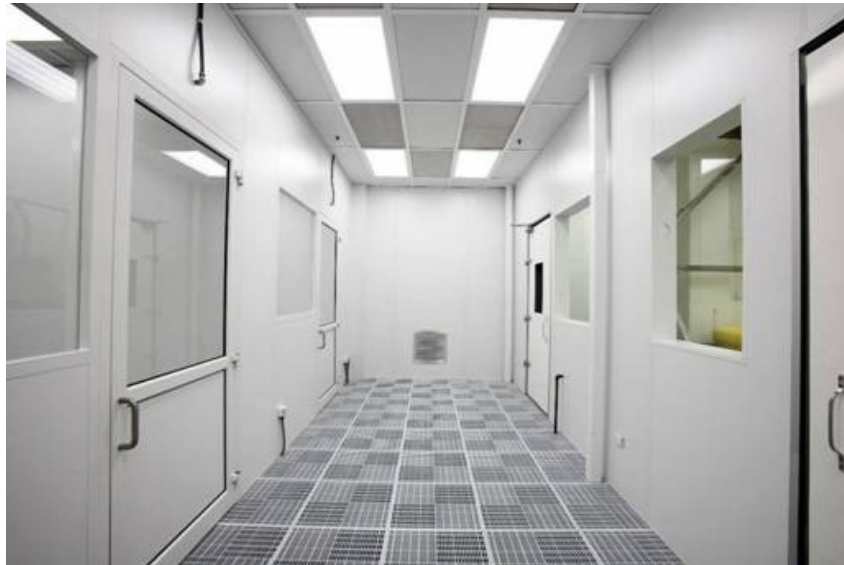
Fig. III-4. The common clean anteroom of the joint ANL/FNAL SCSPF. An additional pair of class-100 clean areas (not shown) lie through the doors to the left of the figure.
