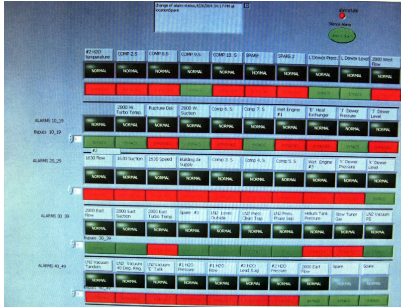
Fig. II-7. The new cryogenic alarm system control screen.
