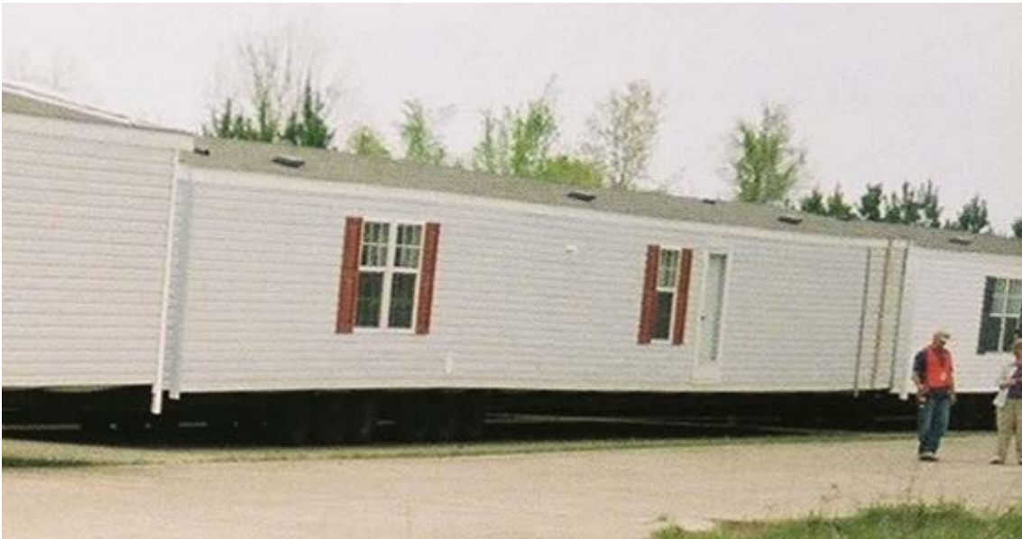
Figure 1 – Example of warped manufactured home at Hope, Arkansas.
