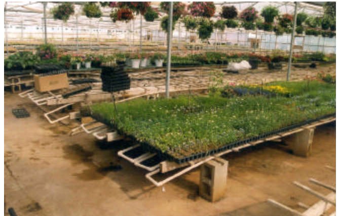
Interior of a greenhouse with the PVC heating pipes under the benches.
