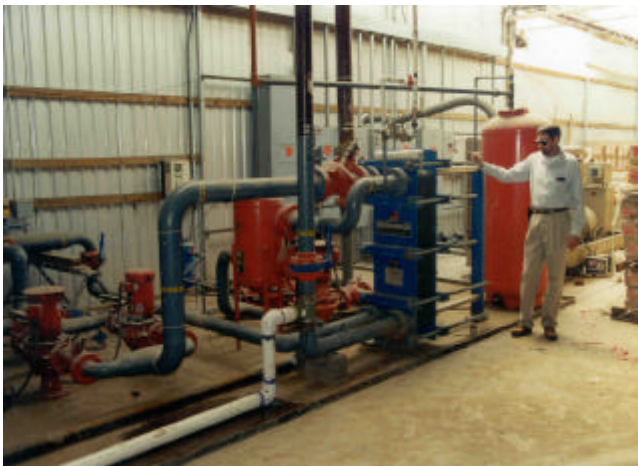
Photo 4. The existing plate heat exchanger (Jim Witcher).
