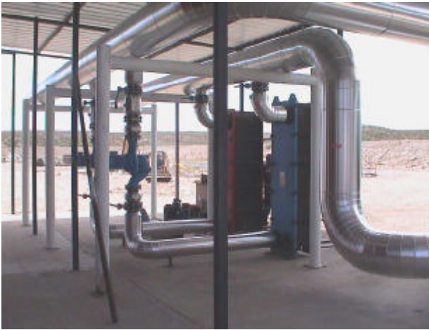
Photo 3. The two new plate heat exchangers.
