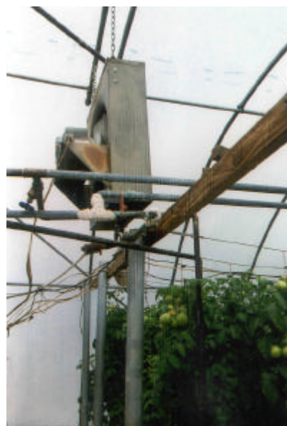
Fan coil heaters at the end of a greenhouse.
