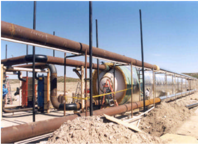
Photo 2. The 167,000-gallon storage tank.
