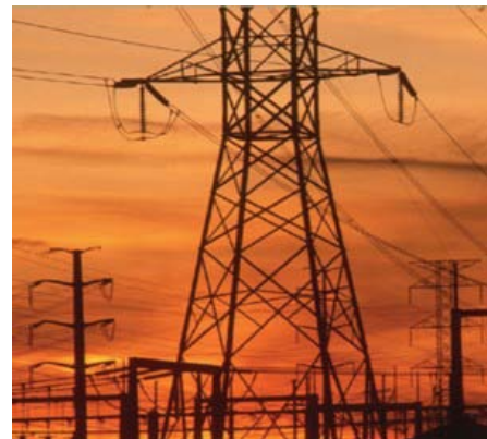
Electricity Transmission Infrastructure
