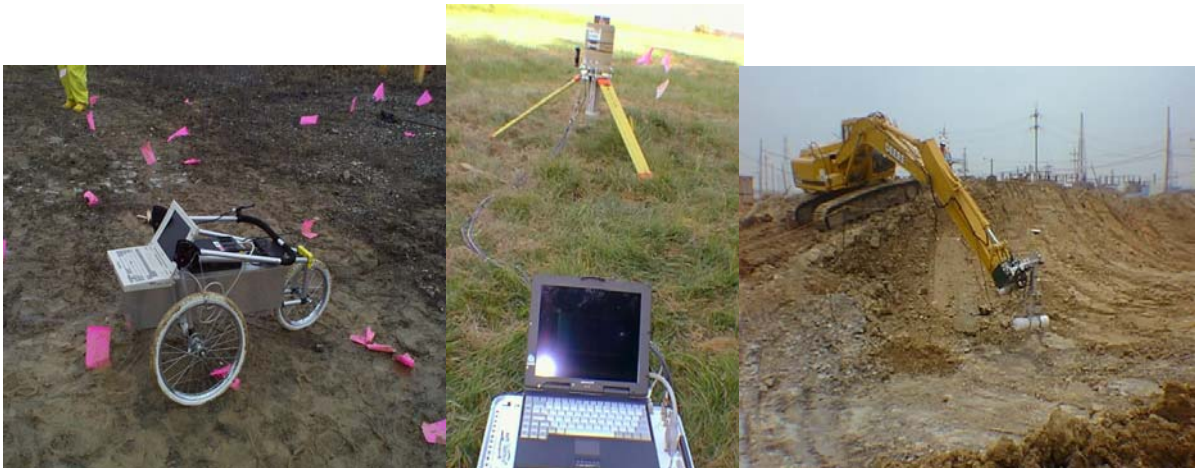
Real-time detection systems include, from left to right, the NaI-based Radiation Scanning System (RSS), tripod-mounted HPGe, and the Excavation Monitoring System (EMS).
