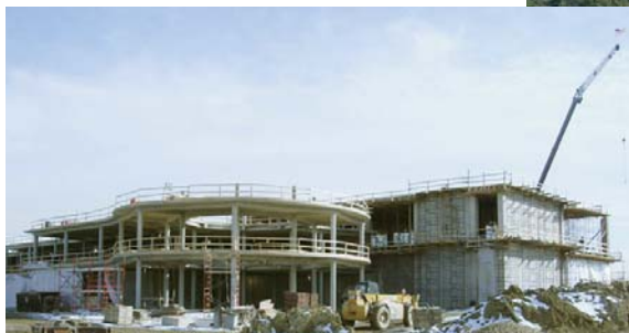
Below: The Center for Nanoscale Materials (as of March 2005), under construction on the west side of the APS experiment hall.
