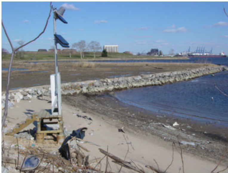
Figure 14. The one-year tide station at Ft. McHenry Wetlands showing the equipment shelter and GOES antenna and solar panel towers.
