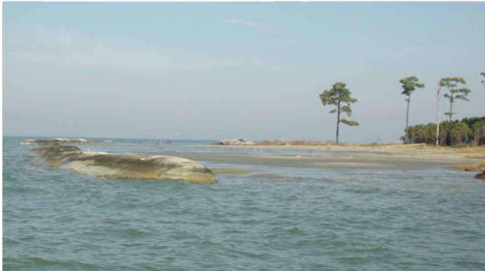
Figure 1. Geotextile tubes placed on the northwest side of Barren Island by USACE retain dredge material used to create new marsh uplands while providing a wave break for the eroding island.
