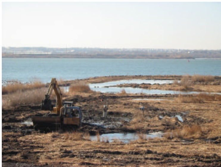
Figure 12. Photograph showing the use of leveling rod to determine depth of one of the ponds being sculpted by the heavy machinery.
