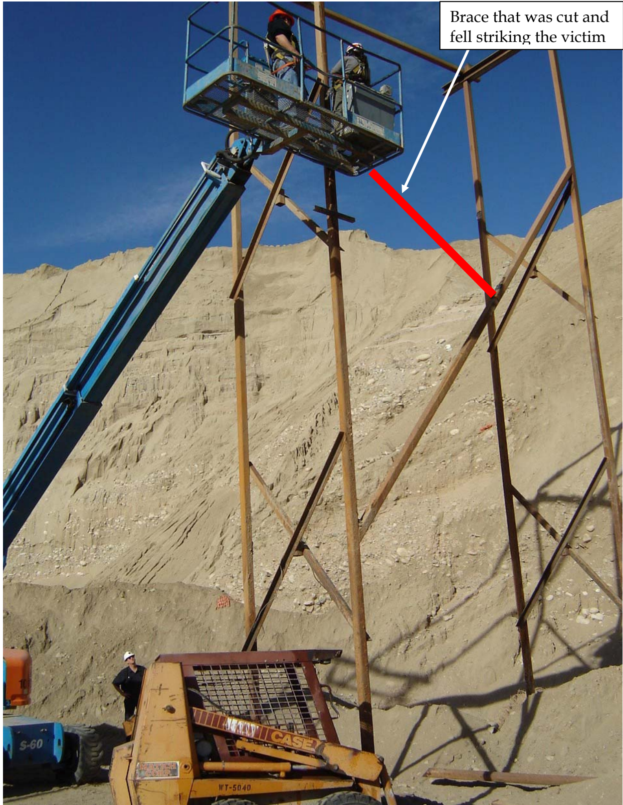
This illustrates the position of the man lift and skid steer loader at the time of the accident.
