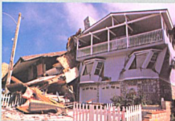
House on left was pushed onto the house at right by the slide. Photograph by Howard Wilshire.
