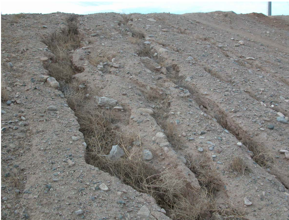
Figure 5.2-2. Gully formation measured over six feet deep in Albuquerque, NM
