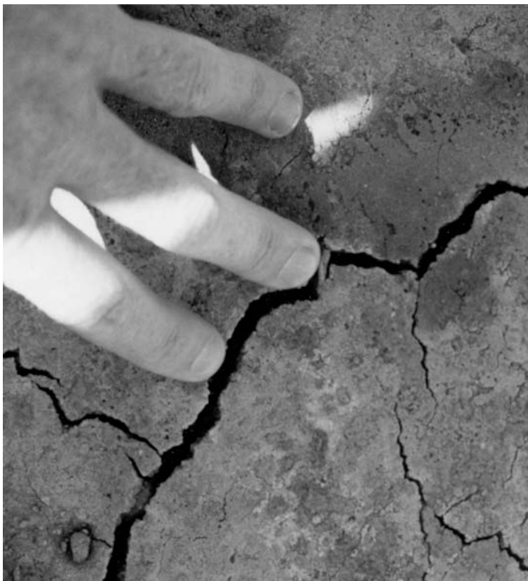
Figure 7.3-3. Desiccation cracking in clay barrier layer
