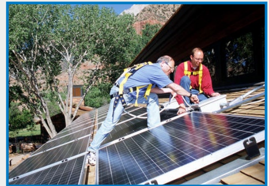
State Implementation Plans (SIPs) encourage energy-efficient building projects, such as applying photovoltaic technologies, to meet air-quality goals.
