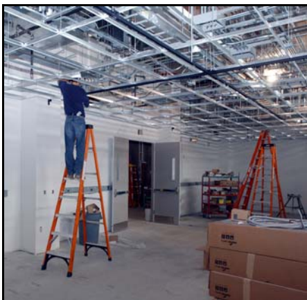
Workers are constructing the research laboratories in the 71,347 sq. ft. multi-level Science and Technology Facility.
