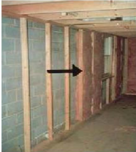
Interior basement insulation with unfaced batts between framing.
