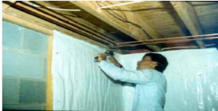
Interior basement insulation with vinyl facing.
