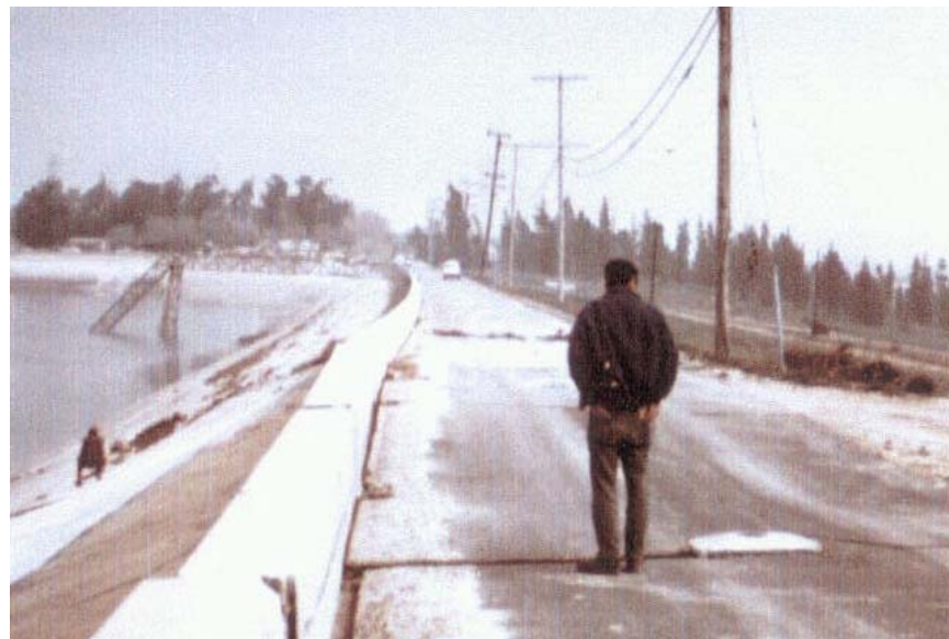
Fig. 2-13 View of Upper San Fernando Dam showing horizontal and vertical deformations and cracks in the upstream face of the dam
