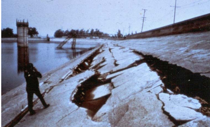
Fig. 2-14 Close-up View of Cracks in the Upstream Face of Upper San Fernando Dam
