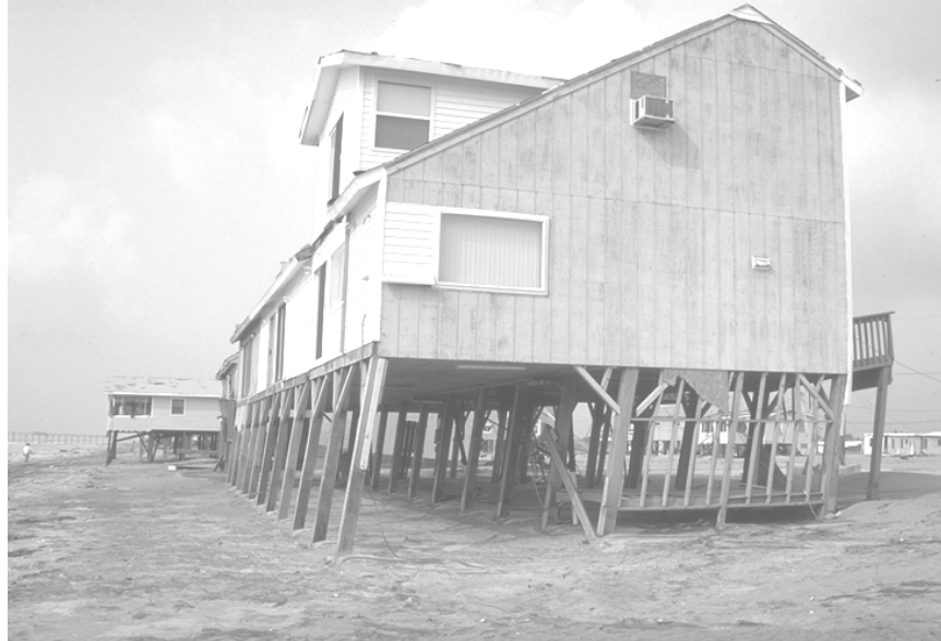
Figure 5-17: This house had inadequate pile embedment and cross bracing
