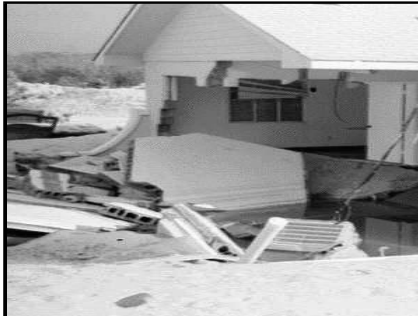
Figure 1-16. Beaches are particularly susceptible to undermining of foundations due to velocity flows.
