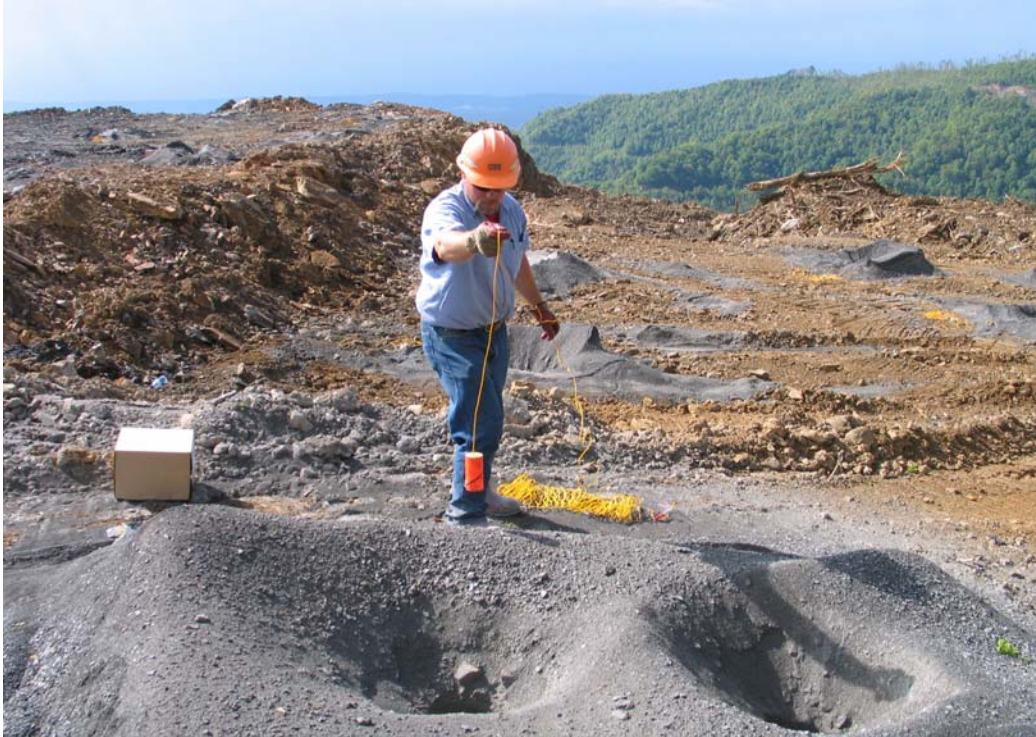
Figure 13 - Priming a blasthole with a booster prior to loading with ANFO-emulsion blasting agent
