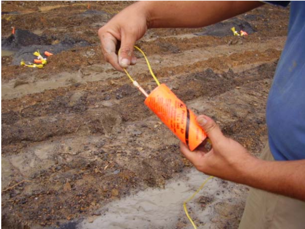
Figure 11 - Preparing a primer by insertion of an electronic detonator (UNI Tronic™ 500) into a booster
