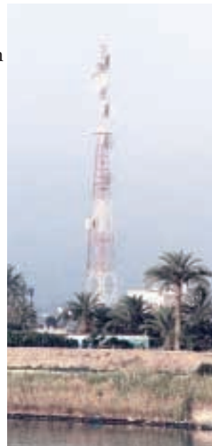
View of a radio relay tower on the west side of the Suez Canal, Egypt.
