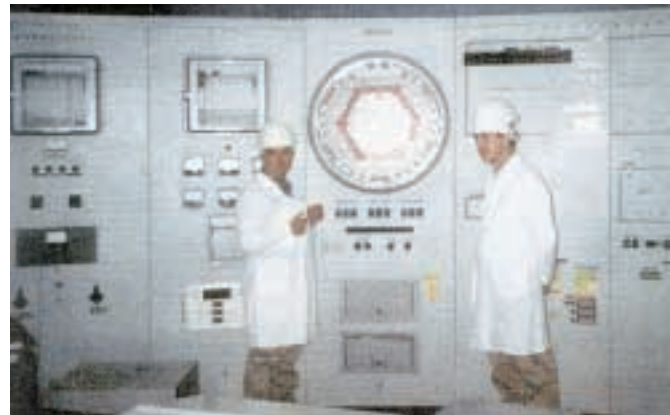
Control center panels for the BN-350 Breeder Reactor at Akhtau, Kazakhstan.
