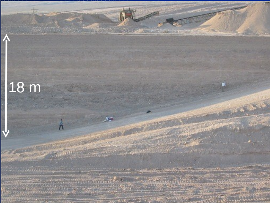
Waste trench under construction – 18 m ... 1/6 th of the way to the water table
