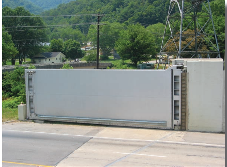
Gate in floodwall, Harlan, KY (photo courtesy of USACE)
