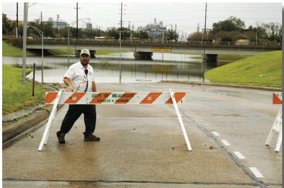
Flooded underpass, Beaumont, TX (photo courtesy of L. Roll/FEMA)
