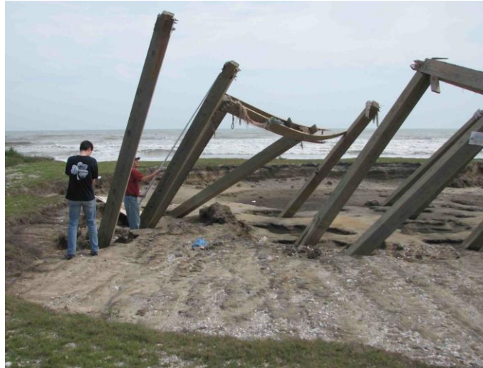
Figure 1. The remains of a Gulf-front home destroyed by Hurricane Ike on the Bolivar Peninsula, Texas. Waves and currents eroded the large depression. The piles tilt in the direction that the waves were propagating (Photo: 3/8/2009).
