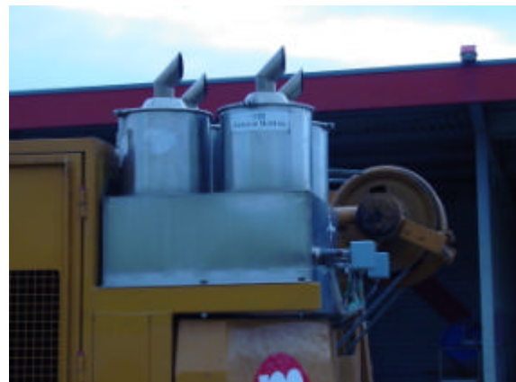
Duplication of Filters increases costs, i.e. on larger, higher horsepower V8 engines. Increases maintenance and repair
