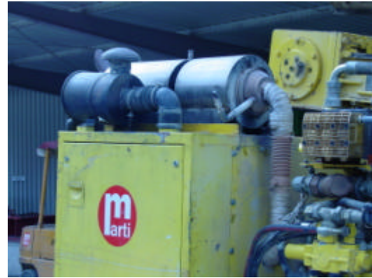
Clobbered installation: long tubing from engine, heat losses, vibration
