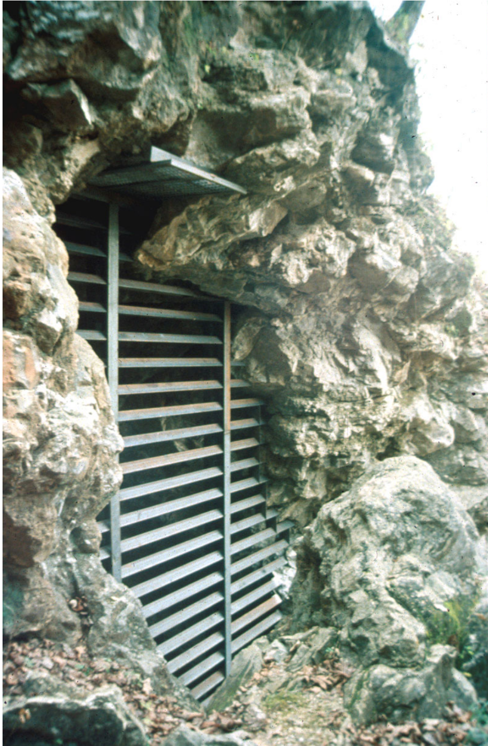
Figure 2. Bat gate installed at Monte Cristo Zinc Mine, Buffalo National River, Arkansas. (1993)
