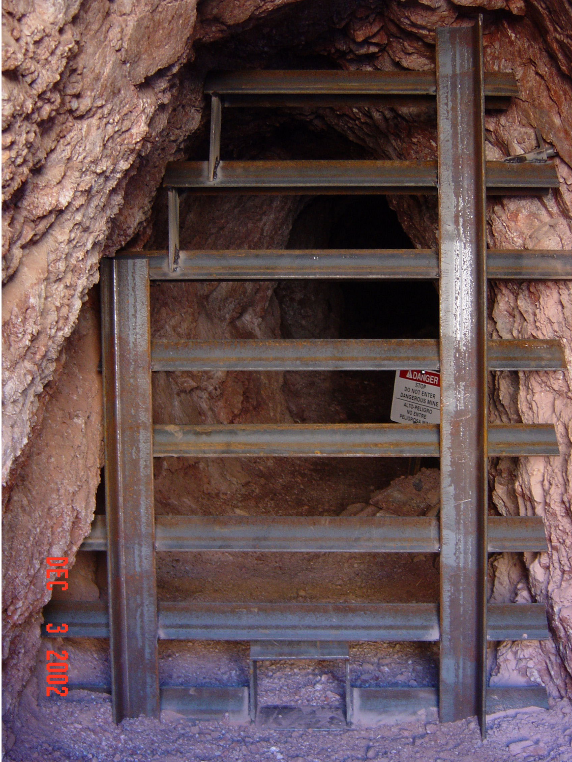
Figure 7. Bat gate at Katherine Access Gold Mine, Lake Mead National Recreation Area, Arizona. (2002) Note special access at base to accommodate desert tortoise, also known to use the mine.
