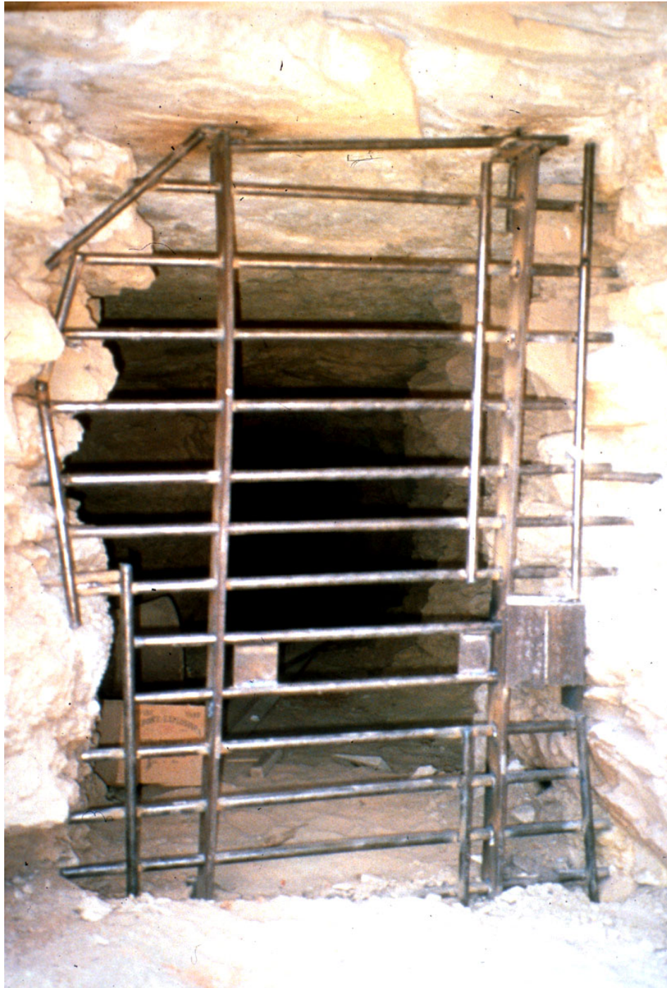
Figure 5. Manganal steel bar bat gate installed at Shafer Uranium Mine, Canyonlands National Park, Utah. (1998) Several perfectly-preserved wooden dynamite boxes dated 1953 were found in the mine, and were left within view of the gated entrance as part of the park's effort to interpret the mining history of the park.
