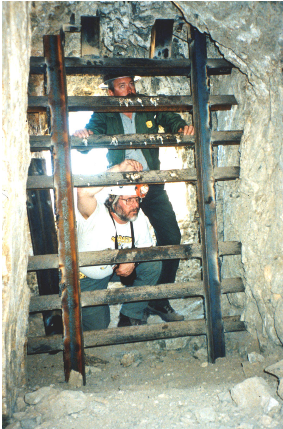
Figure 6. Inspecting bat gate at Sullivan Gold Mine, Joshua Tree National Park, California. (1999) Middle bar removed for access.
