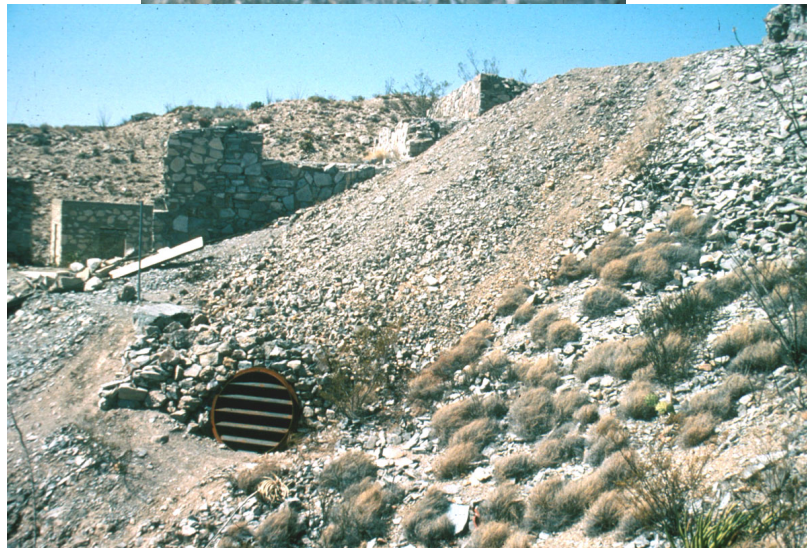
Completed bat gates at Mariscal Mercury Mine in Big Bend National Park. Note protective lock box for removable bar locking mechanism, and culvert gate used to maintain opening on unstable slope. This project was funded and contracted by the Railroad Commission of Texas Division of Surface Mining and Reclamation.
