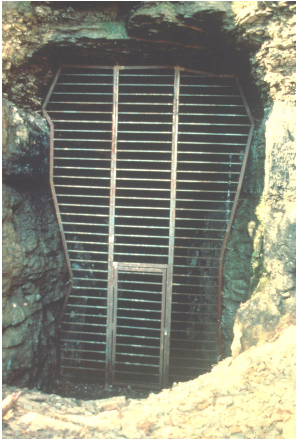
Figure 1. Bat gate installed at Kaymoor Coal Mine, New River Gorge, West Virginia. (1988)
