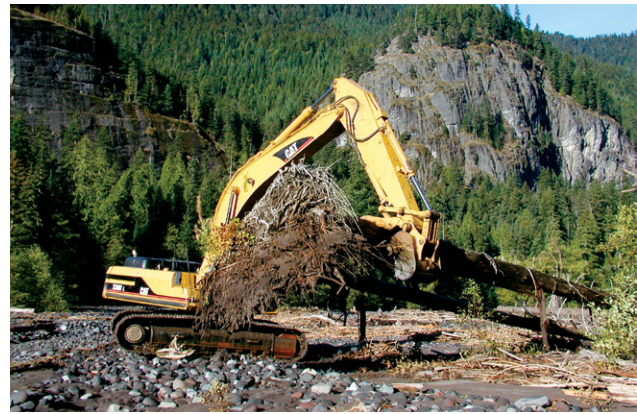
Don't try this at home! At Mount Rainier, construction of emergency engineered log jam to reduce flood damage in a fish-friendly manner. (Paul Kennard)
