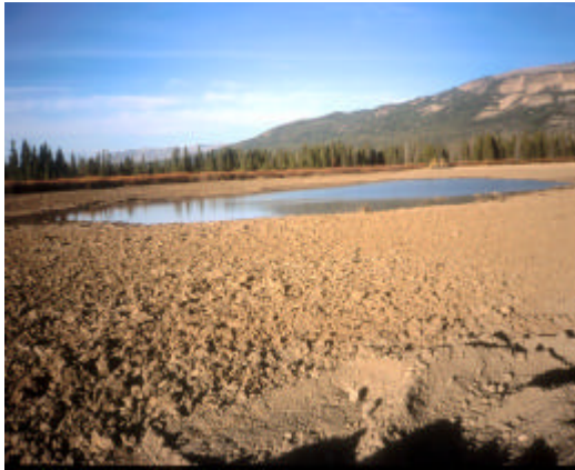
Final grading was completed by the end of October 2002. Steep-walled borrow ponds were reshaped into river oxbow features, and mine waste was removed to form wetland and riparian communities. Planting will occur in spring and early summer of 2003.
