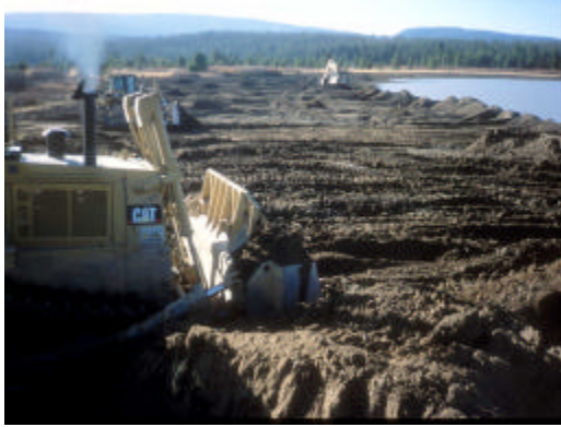
Contractors moved over 350,000 cubic yards of earth to create the pond shoreline configurations and wetland and riparian zone elevations called for in the design.
