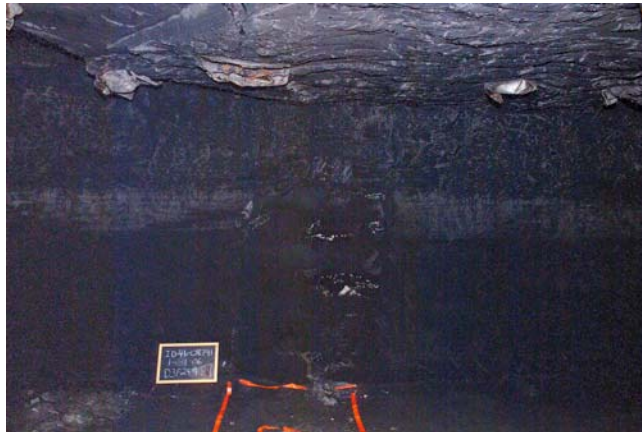
Figure 24 - Post-Explosion Location of Seal No. 5
