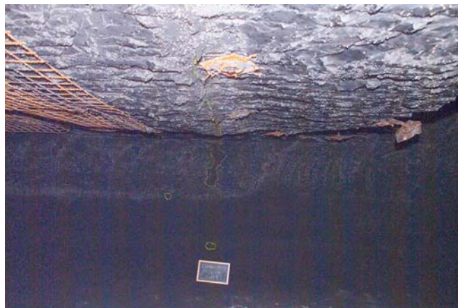
Figure 26 - Post Explosion Location of Seal No. 7
