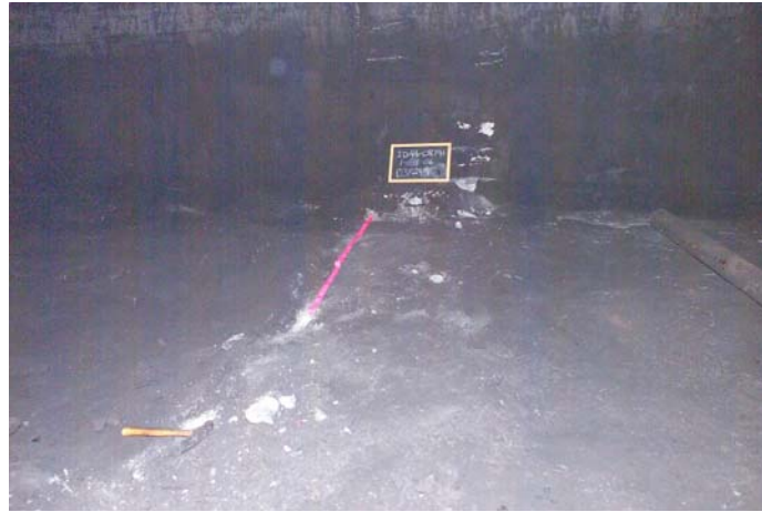
Figure 25 - Post-Explosion Location of Seal No. 6
