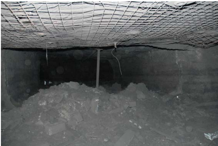
Figure 6 - Damaged Stopping at 59 Crosscut, No. 4 Belt
