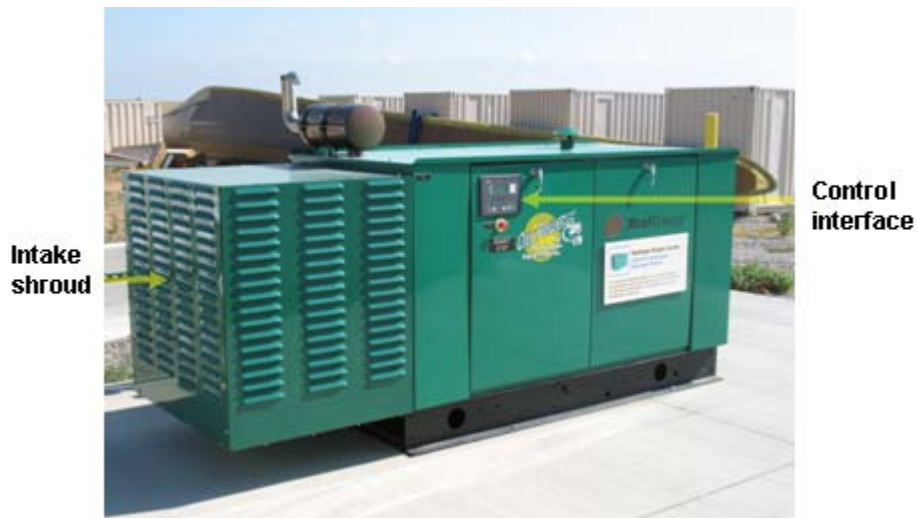
Figure 2-11: Hydrogen-fueled internal-combustion generator
