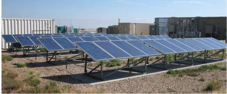
Figure 2-12: 5 kW east PV array at NREL’s DERTF
