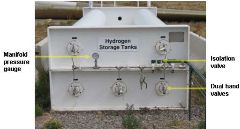
Figure 2-10: Hydrogen storage tanks
