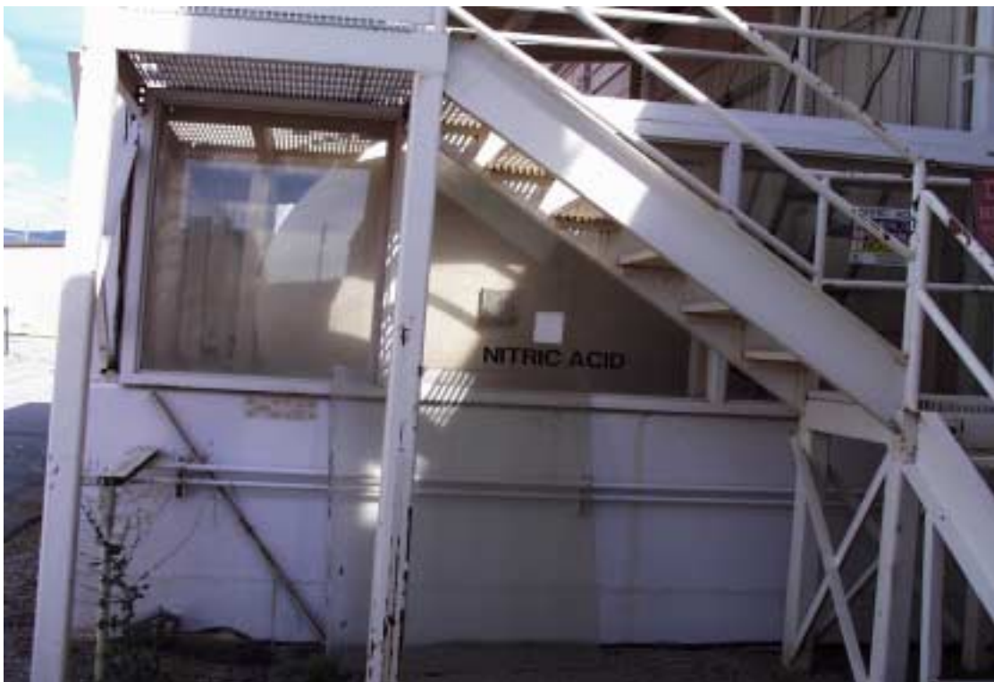
Figure 7-1. Nitric Acid Tank.
