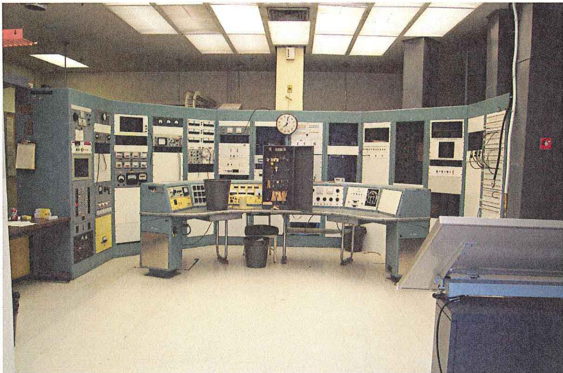
Figure 4. Van de Graaff Accelerator Control Room
