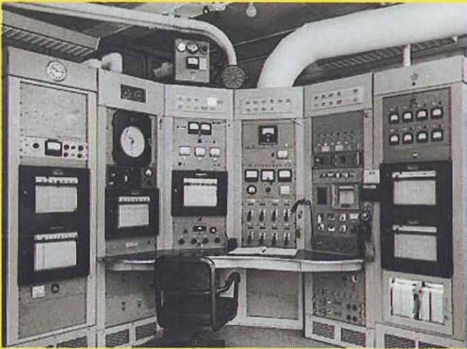
OWR Control Panel
