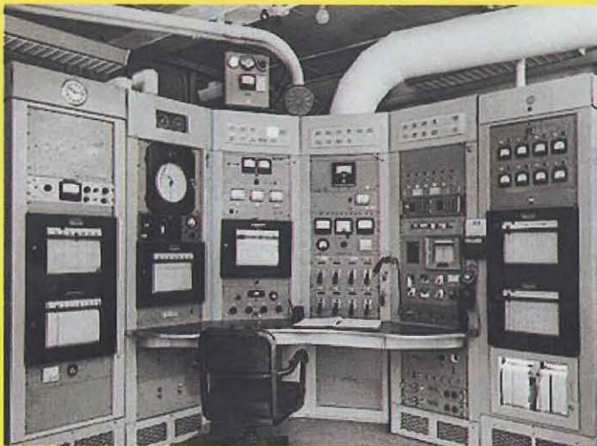
OWR Control Panel
