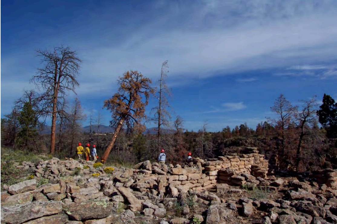
Figure 20.1. Snag removal at Nake'muu to decrease risk of possible damage to standing walls.
