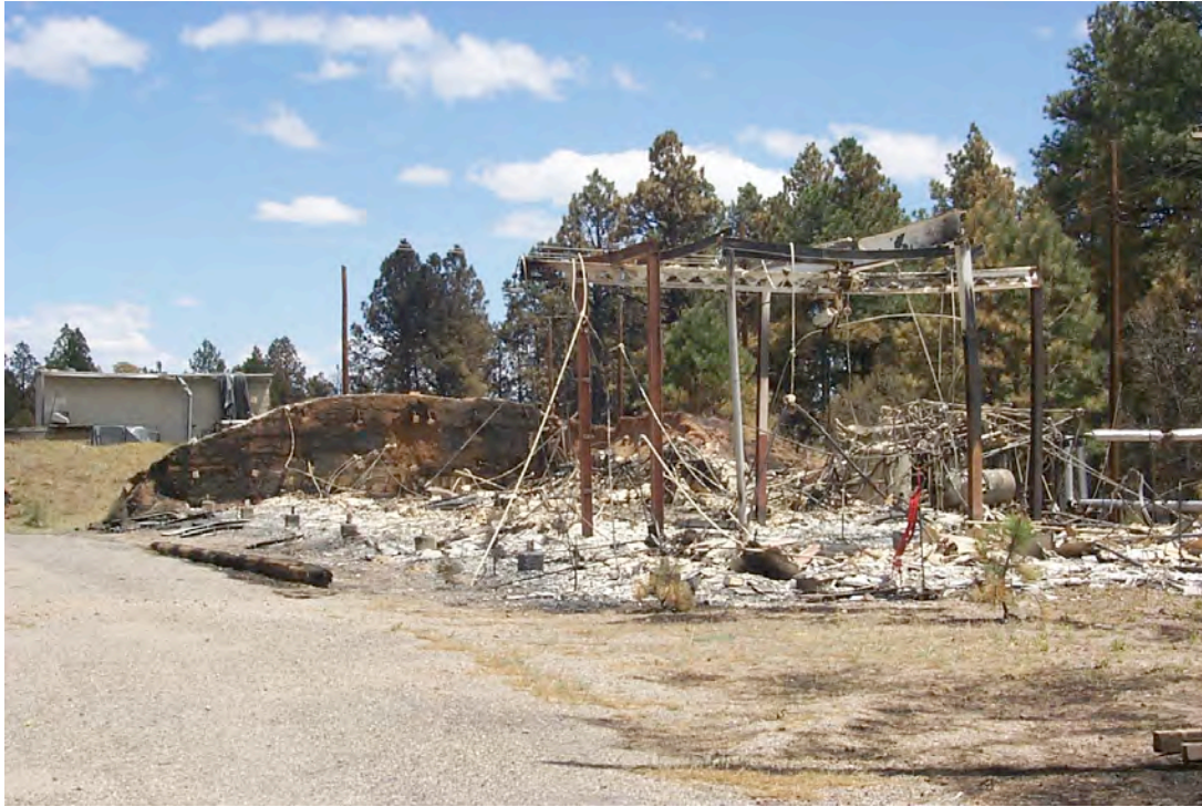
Figure 15.3. The same buildings as in Figure 15.2 after the Cerro Grande fire.
