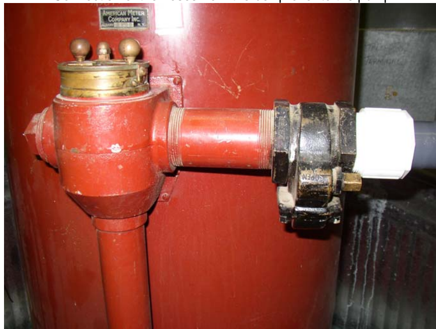
Valves on Bell Prover.
