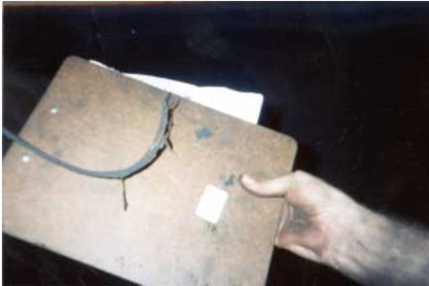
Figure 29: Located near the inby left corner at spad #13348. Picture of melted insulation jacket of phone cable.
