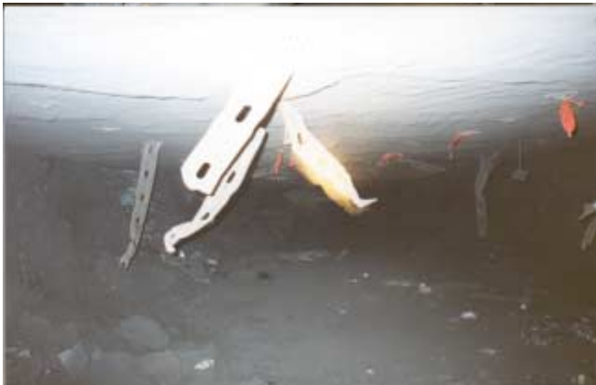
Figure 7: Metal channels shredded and torn in the last open crosscut between #2 and #3 entry. Looking from the #2 side approximately 20 feet into the crosscut. The red flagging indicates loose roof bolt plates.
