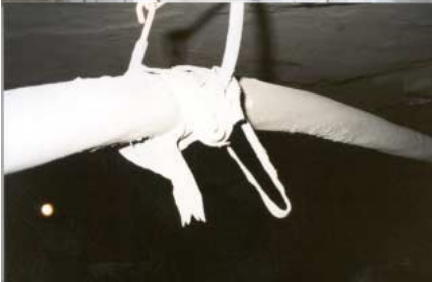
Figure 26: Located at the left outby rib corner at spad #13231 in the #2 entry. Picture is of a “J”hook and shielding melted into high voltage cable.
