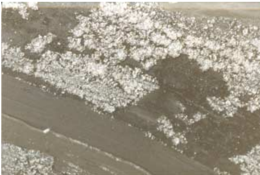
Figure 35: Picture of coking on the roof starting 30 feet outby the #3 face.
