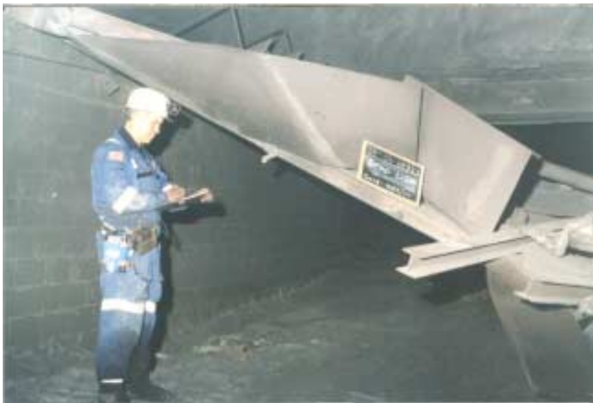
Figure 22: Looking outby at spad #12285. Picture shows damaged vercast.
