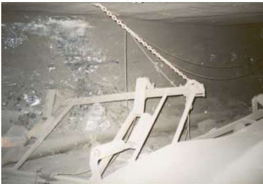
Figure 13: Looking into the #3 entry from the crosscut located between spads #13296 and #13300. Damage to the conveyor belt system increased outby.
