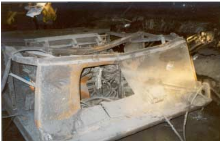
Figure 6: No. 4 section belt power center. Taken from the #3 entry side at spad #13207.
