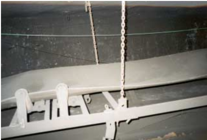
Figure 12: Beltline looking into the #3 entry from the crosscut located between spads #13313 and 13314.
