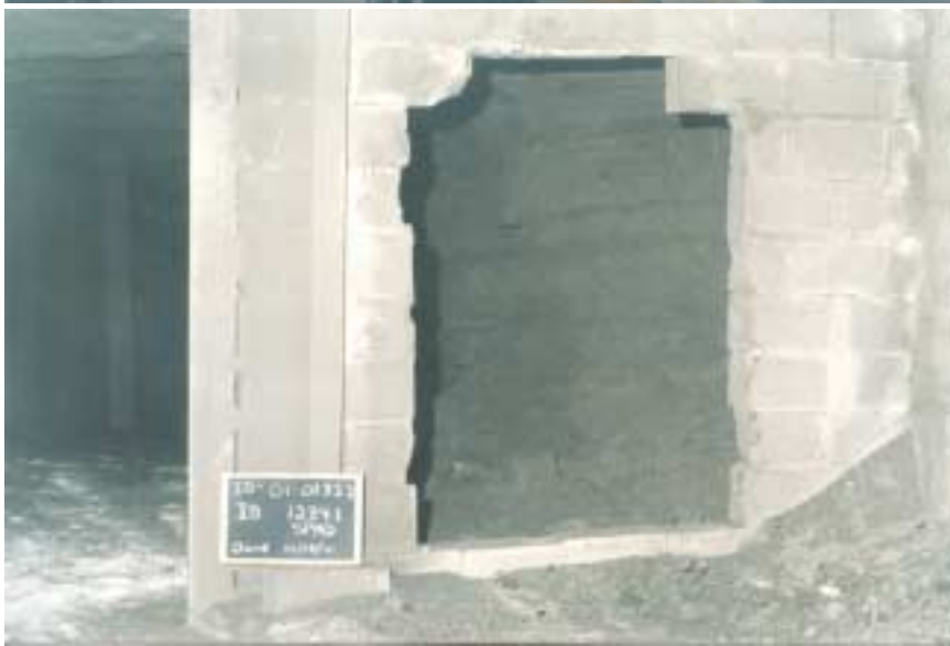
Figure 21: Looking outby toward spad #12341, located in the #1 entry of 3-east. This picture shows damage to 3-east return regulator.
