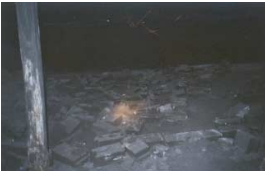
Figure 1: Concrete block blown from a stopping between #1 and #2 entry, taken from the #2 entry at spad #13295.
