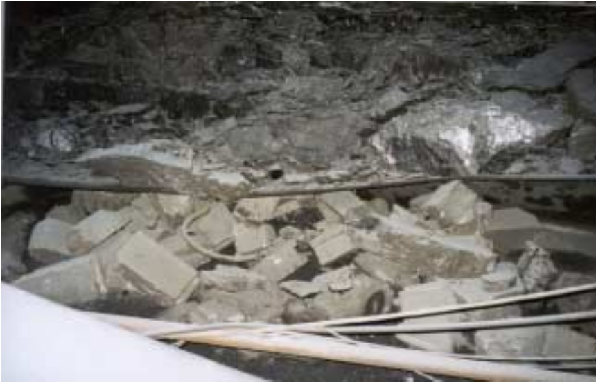
Figure 17: Looking into the #3 entry from the crosscut between spads #13200 and #13199. Stopping material along with the damaged conveyor belt system deposited along the left rib in the #3 entry can be seen.
