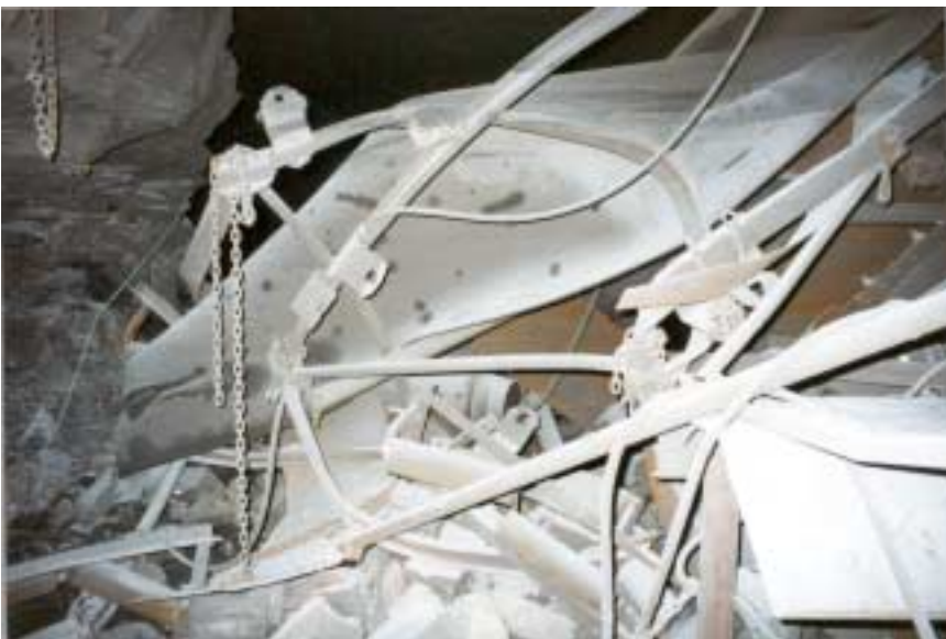
Figure 19: Taken from the left of spad #13038 looking in by into the #3 entry of the left ribline at the No. 4 section header. Concrete blocks from the inby overcast can be seen at the bottom of the picture.
