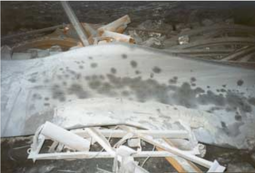
Figure 18: Looking into the #3 entry from the crosscut between spads #13039 and #13048. The steel beams, steel plates, and concrete blocks from the belt/return overcast along with material from the conveyor belt system were deposited along the left ribline of #3 entry. Note: In the upper portion of the picture the steel beams from this overcast can be seen twisted and bent.
