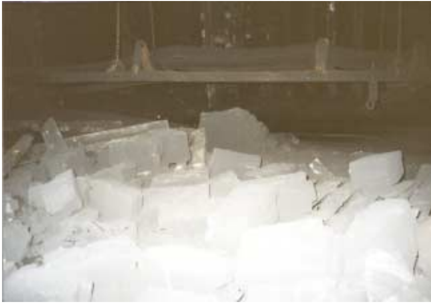
Figure 11: Stopping material deposited in close proximity to where they were originally built. The upper portion of the picture shows the conveyor belt system. This picture was taken from the #4 entry looking into the #3 entry at the crosscut inby spads #13320 and 13318. The picture indicates very little damage to the conveyor belt system.
