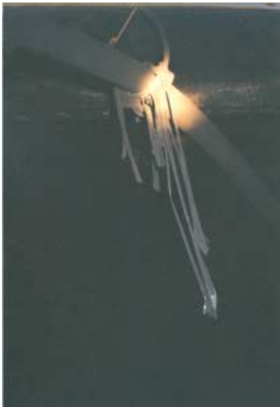
Figure 27: Located along the left rib of #2 entry at spad #13319. Picture of melted shielding hanging off high voltage cable.
