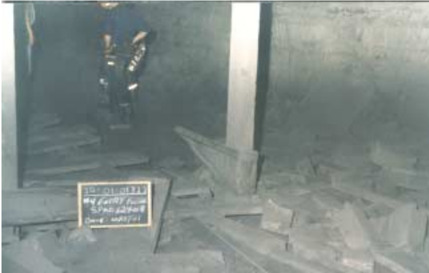
Figure 23: Looking outby at spad #12408. Picture shows the position of a metal panel from a metal stopping.
