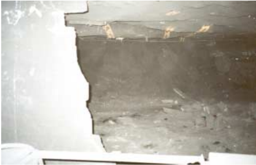
Figure 2: Partial concrete block stopping behind the section power center looking toward the #1 entry.
