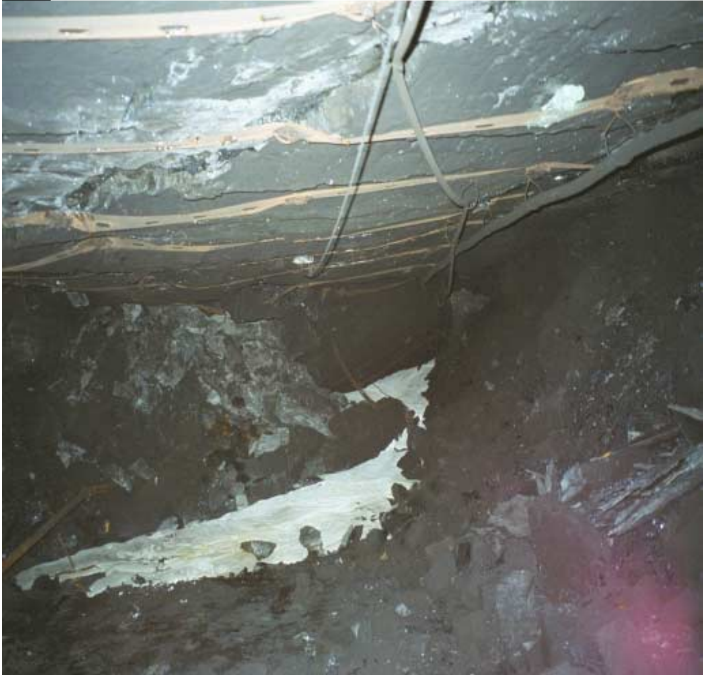
This picture was taken facing outby at Spad #13348 in the # 2 entry toward the rockfall at Spad #13333. A well-defined joint/slip can be seen in the roof. The roof straps and roof bolt plates can be seen across the joint/slip running diagonal from right to left. This is a clear indicator that this well-defined joint/slip was present at the time of the roof bolt installation.
