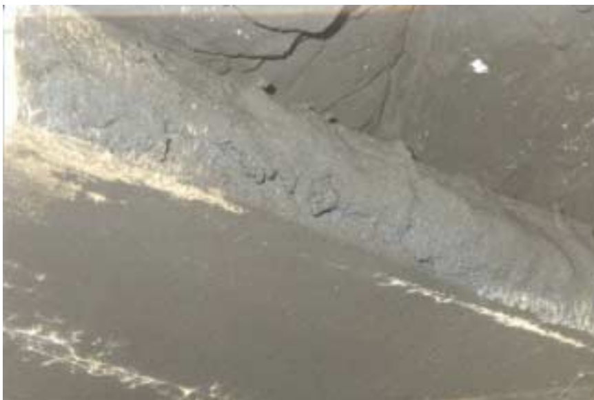
Figure 32: Located in the last open crosscut between spad #13352 (#2 entry) and spad #13353 (#3 entry), 50 feet into the crosscut from #3 side. Picture of coking on “T-Board”.
