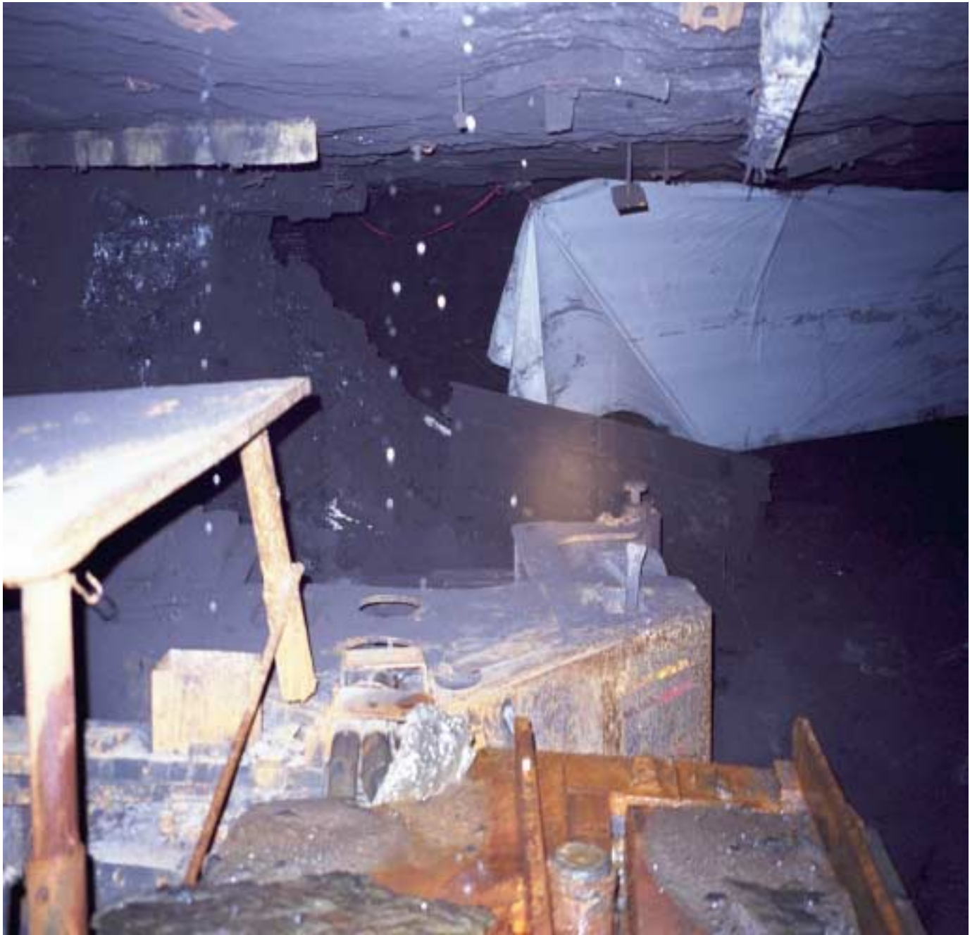
The roof of the crosscut above the scoop between Spad 13352 in the #2 entry is shown without any straps installed. This was evident in all the crosscuts between # 1and # 2 entries even when the slips and joints were well-defined in the roof of the crosscuts.
