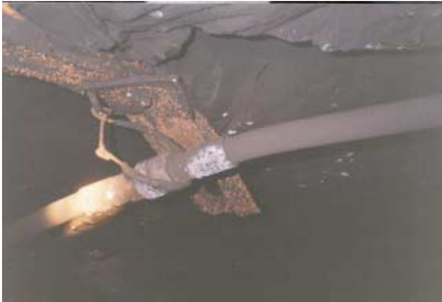
Figure 30: Located in the #1 entry inby spad #13349 along the right rib. Picture of a melted “J” hook on the continuous miner water line.
