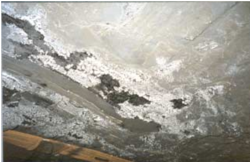
Figure 34: Located in the #3 entry inby the last open crosscut (Inby spad #13353). Picture of coking on the roof starting 30 feet outby the #3 face.
