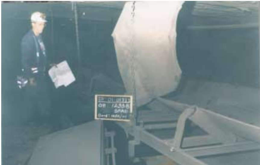
Figure 20: Looking outby from spad #12338, located in the #3 conveyor belt entry of 3-east. A piece of a belt vulcanizer is blown into belt structure. This picture also shows how the conveyor belt system at this location was only slightly damaged.
