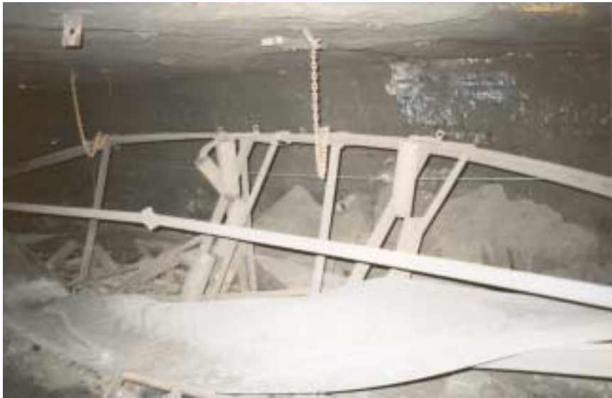
Figure14: Looking into the #3 entry from the crosscut between #3 and #4 entry, to the right of spad #13233. Conveyor belt system is totally destroyed and deposited along the left rib of #3 entry.
