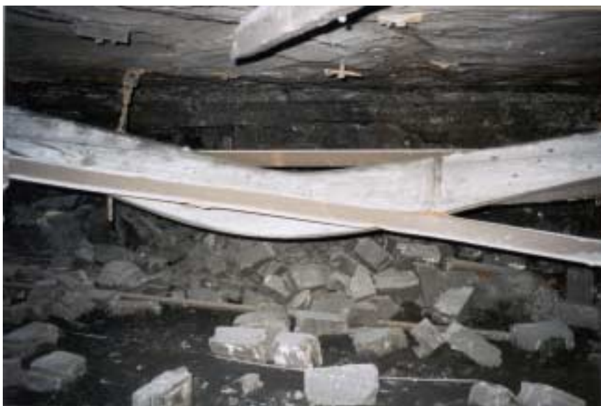
Figure 16: Looking into the #3 entry from the crosscut located between spads #13205 and #13206 stopping material deposited along the left rib of #3 entry. Note: Starting at the outby corner at spad #13206 and extending inby toward spad #13209 in the #4 entry, six broken roof straps were located along the left side of the entry.
