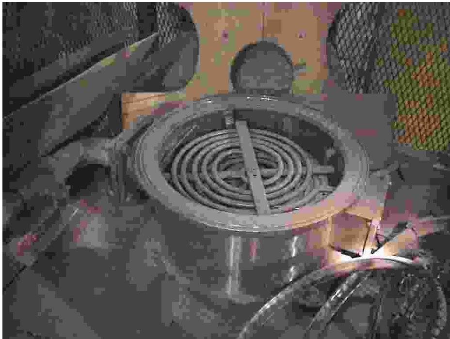
Figure 3. Active Regeneration Station at Deep Post Mine.
